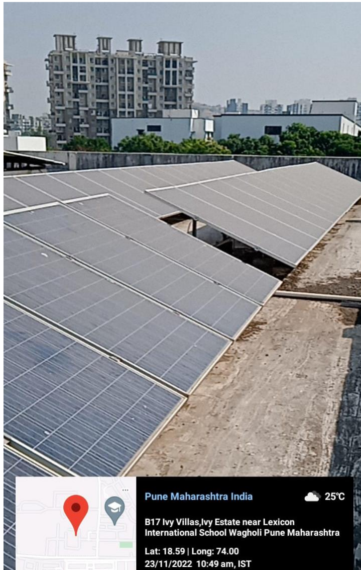
Fig. 1 Solar panle on roof of building-C
