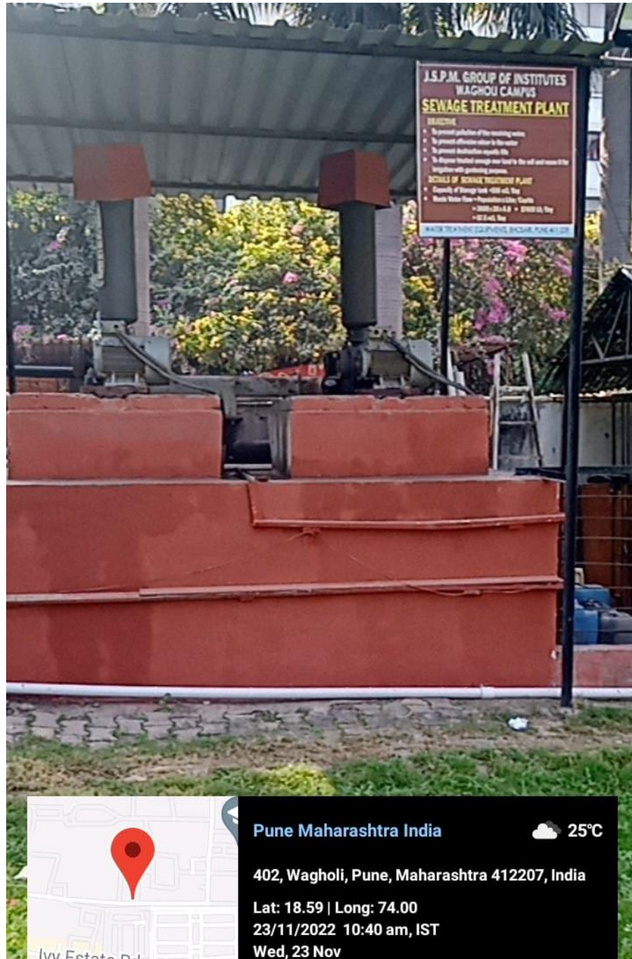
Fig. 7 Sewage Treatment Plant at ICOER
